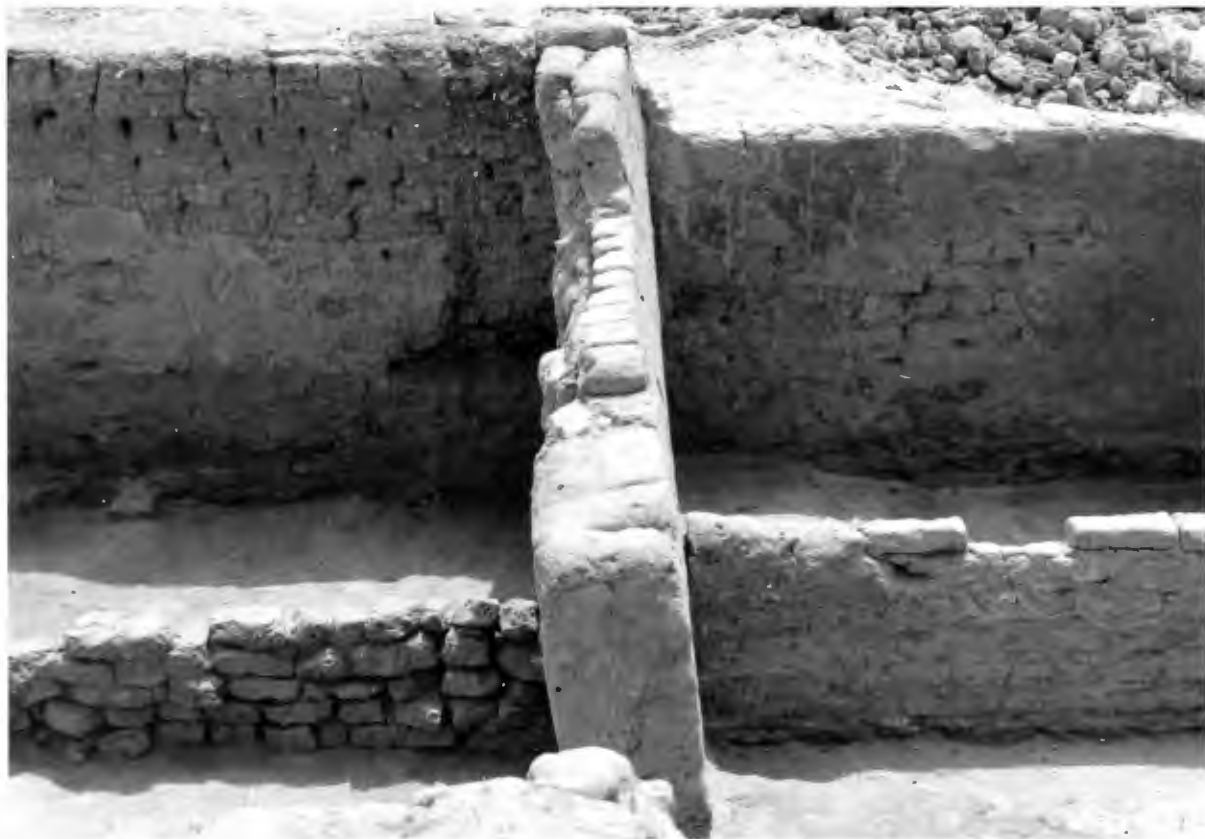
Figure 3.2. The dividing wall between the Front and Middle Rooms, looking south and showing the batter. Note the dividing wall in the Front Room with rounded top at the left end (original access ?), and the rubble wall in the Middle Room.
